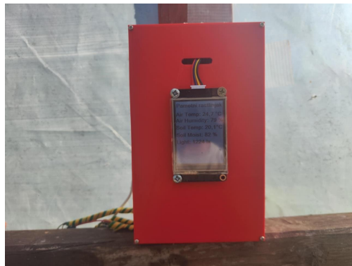
Figure 15: Installed HMI display on the control system enclosure
